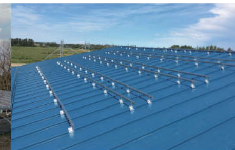
Metal Roof Solar Mount
