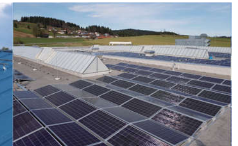
Flat Concrete Roof Solar Mount
